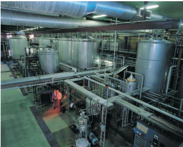
... cooling water systems for power plants, food processing industry, in gas and drinking-water supply lines ...
